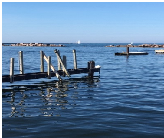
View of a large gap in the breakwater seen from the South Shore finger piers.
